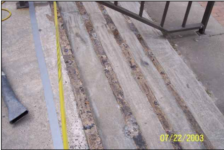
Broken & Worn with the failing nose treads removed.
