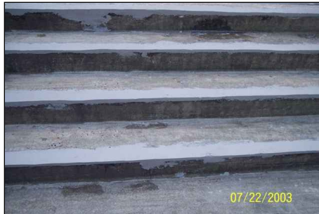
Belzona 4111 (light color) repairs the worn and broken steps awaiting the non slip system
